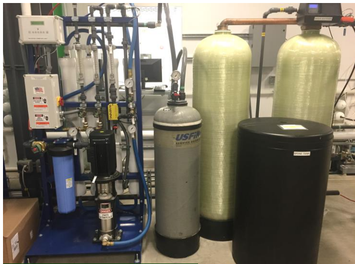
Reverse osmosis system
