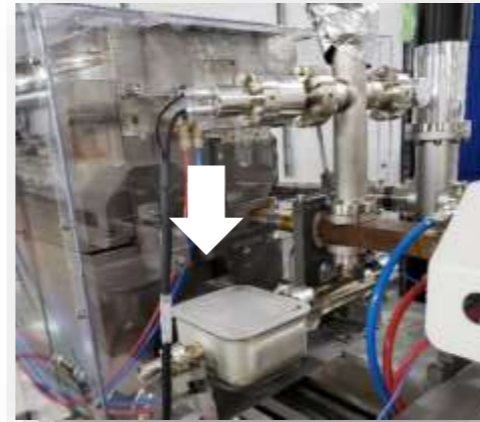
SR ion pump: short-circuit (1 units)
