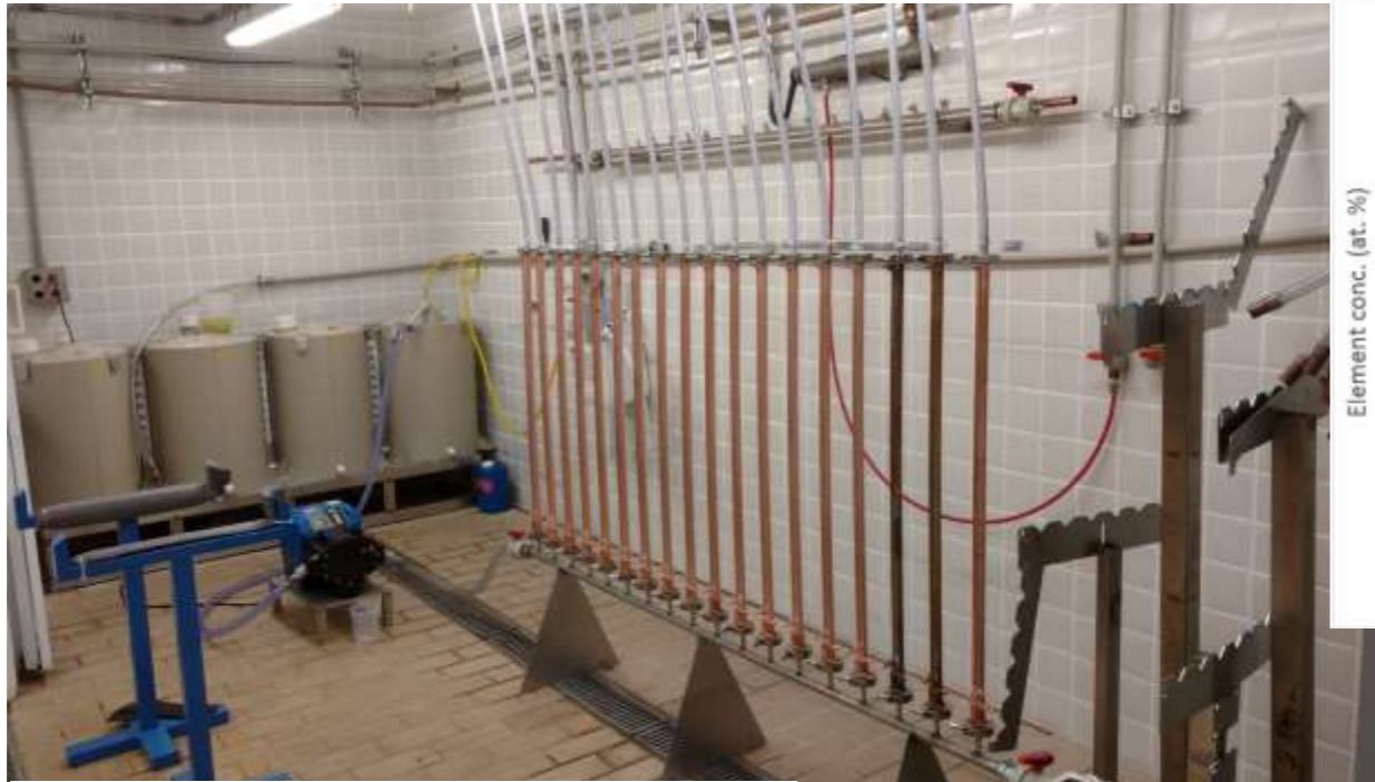
Cleaning facility – recirculation system
