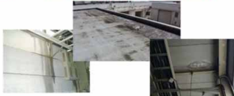
Water leak of MR power supply building
