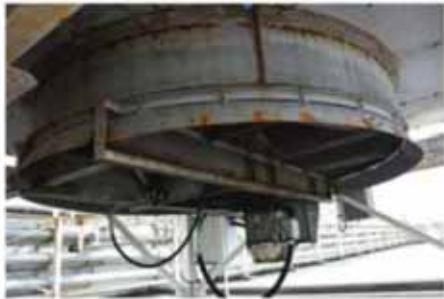
Corrosion of cooling fan for RF system
