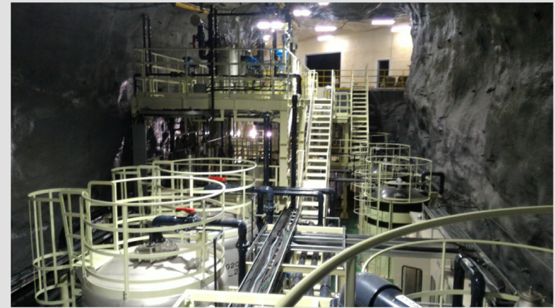
Super-K Gd water system installed in a new underground hall
