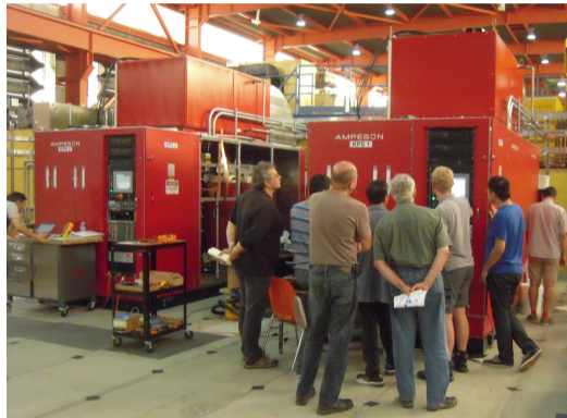
Klystrons' 600 kW 65 kV power supplies (Ampegon) on the e-hall roof
