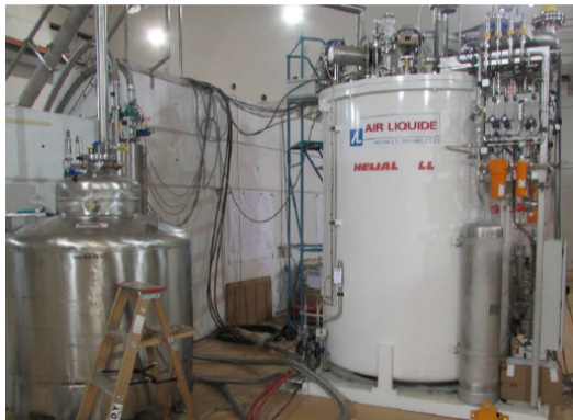
ALAT LL Cold Box, KAESER (FSD571SFC) main compressor (112g/s), Cryotherm - distribution
