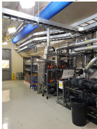
Radon filter system
