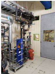
Chilled water loop
