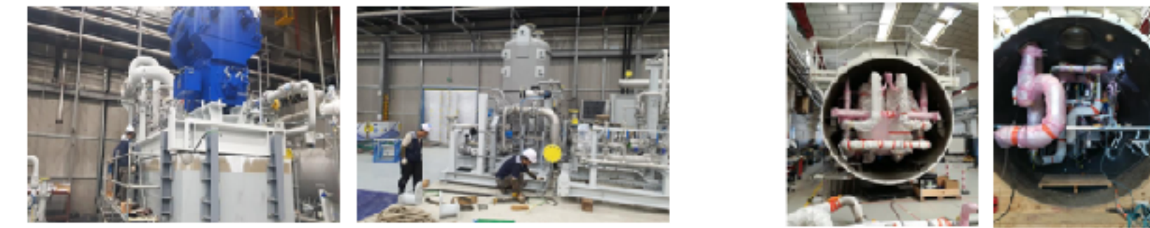
Compressors and Oil Removal System (WCS)
