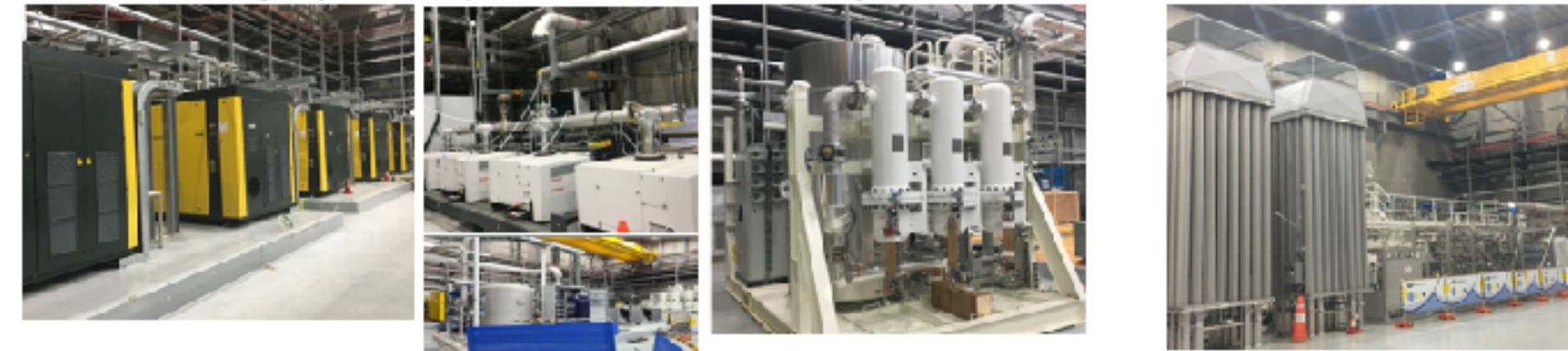
Compressors and Oil Removal System (WCS)
