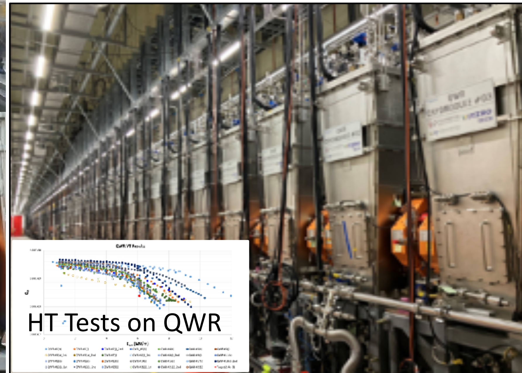
SCL3 LINAC installed on 2021
