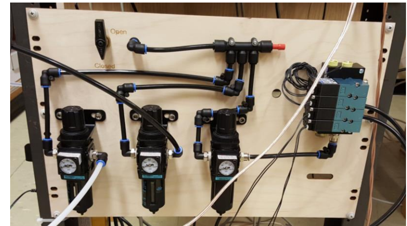
Compressed air gas panel
