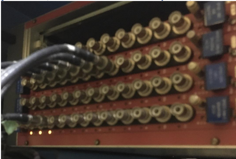
Figure 3: The back of the HV power supply.
