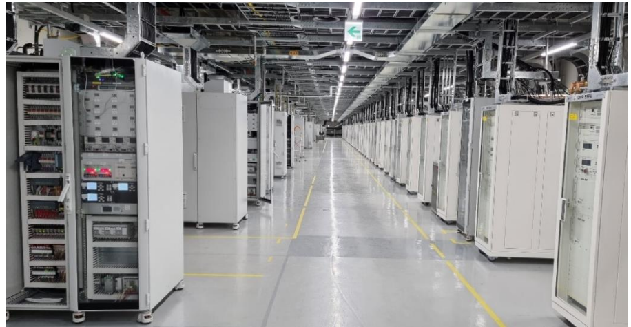
CM/Cryogenic Control Rack and SSPA
