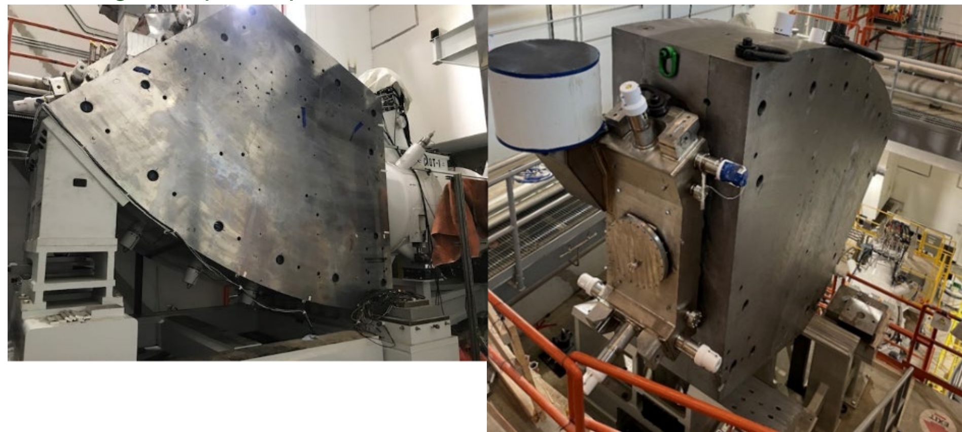
SCD3 magnet (left) and SCD4 magnet (right) installed in vertical preseparator
