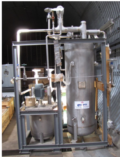
Filter skid (MicroBooNE design): 4A molecular sieve material to remove water contamination and Cu Alumina to remove oxygen contamination. Ten ton LAr recirculation turn over time of ~three hours.
