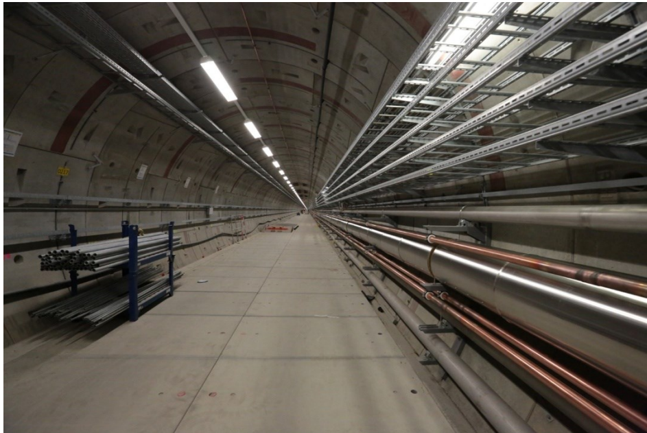
Utilities installed in accelerator tunnel
