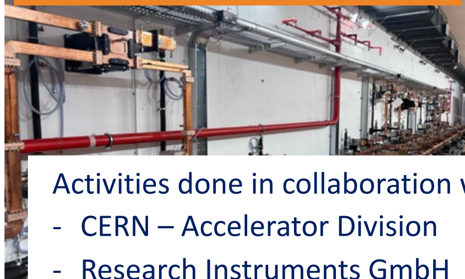
Accelerating structures in Accelerator Bay 2
