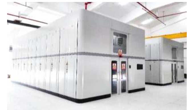
Dipole power supply
