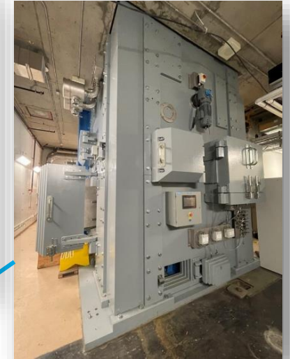
Hot cell facilities consisting of maintenance cell and target disposal cell
