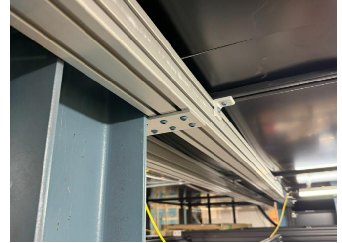
New extrusions on the ceiling
