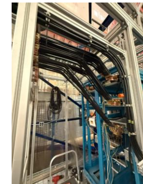
Power-supply connection to the trap
